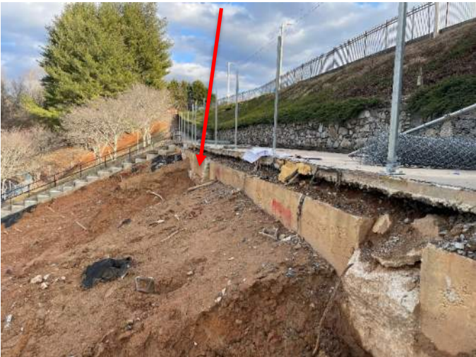
^ Arrow indicates significant foundation undercut erosion with a potential existing grout repair below footing
