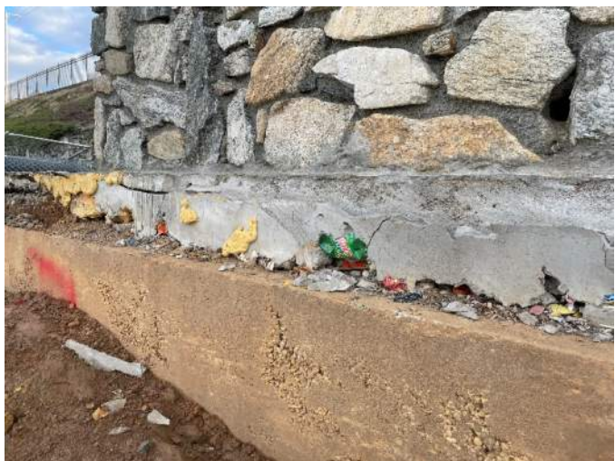
^ Sloppy crack infill between pre-cast and upper concourse
