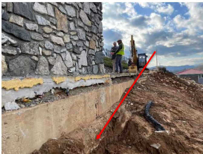
^ Sloppy Infill – exposed footing to be covered
