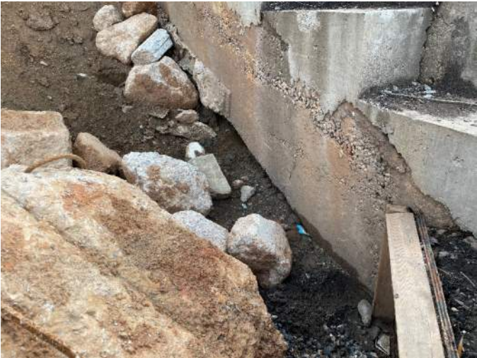
^ Eroded undermining at west raker beam / retaining wall
