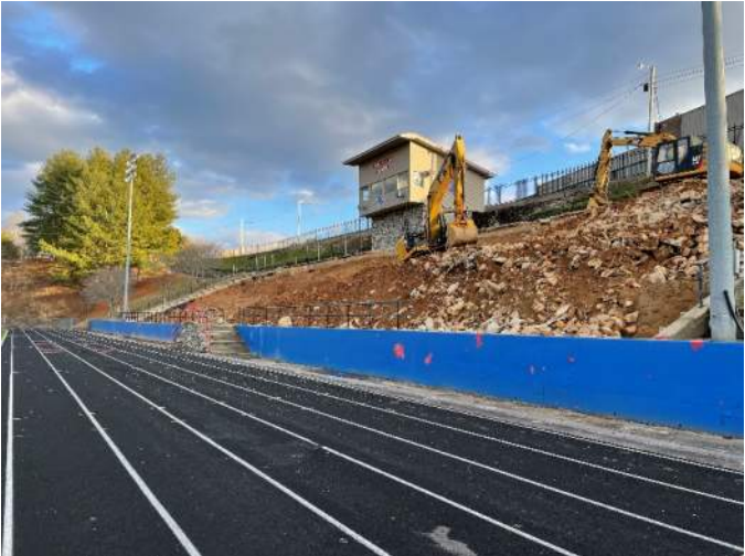
^ Overall homeside demolition view – existing rock steps to be demolished as well
